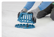
Roof drain systems
